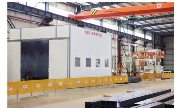
Automated Paint Spraying Room
